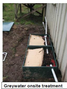
Greywater onsite treatment
