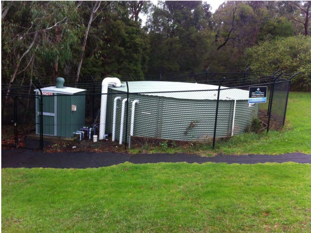
Figure 7 Example Recycled Water Storage Tank
