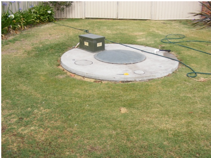
FIGURE 3-6 ONE OF TWO AERATED WASTEWATER TREATMENT SYSTEMS (AWTS) IN THE STUDY AREA
